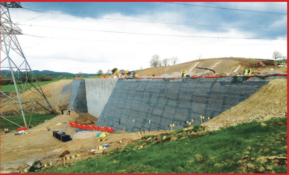
Cumbria Electric sub-station - Old Hutton, UK
