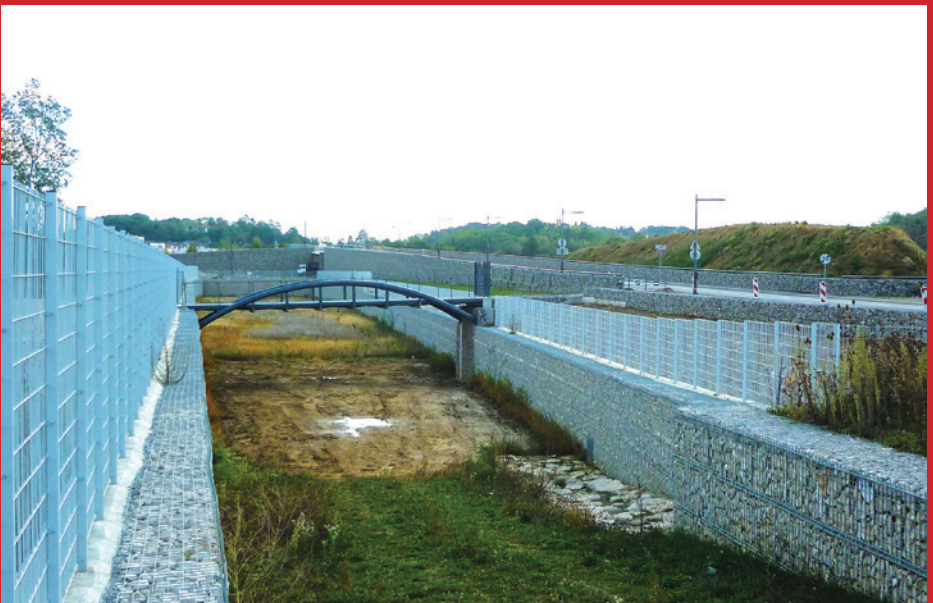
Storm water basin - Decines, France
